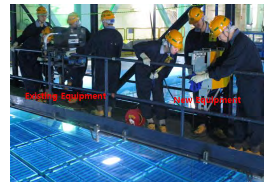
Field experiments were conducted at the Wolsung Nuclear Power Plant to assess the need for an additional optical fiber cable using both existing and newly developed instruments.
